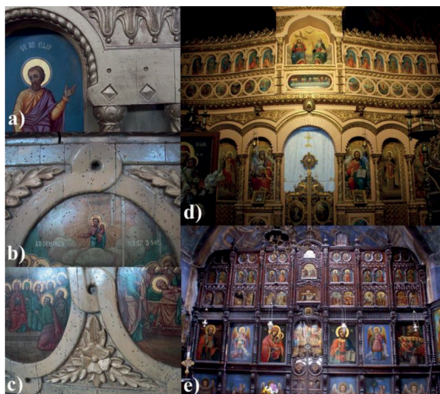
Figure 6.6: Iconostases from Izvoarele churches in Dambovitza county, Southern Romania: a), b) and c) details of parts of the iconostases, showing marks (holes) due to woodworm attack; d) and e) iconostases of the two churches after their complete restoration.
