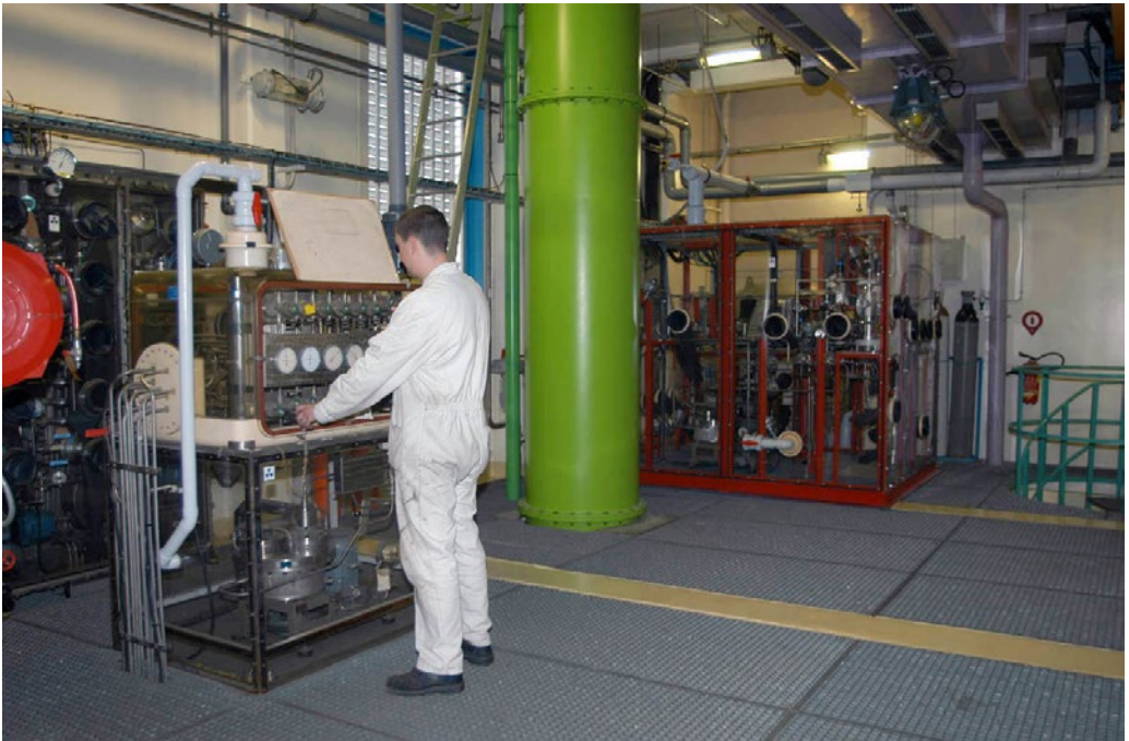
Fig. 5.7: The detritiation facility in 2004. On the left the monitor circuit and in the background the exhaust circuit for the tritium gas.
