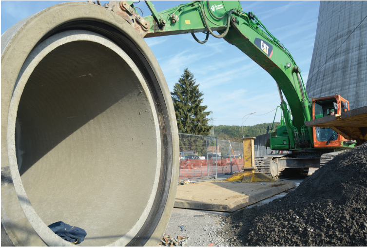
Figure 37.3. Diverting the municipal culvert upstream of the Tihange site. Tihange nuclear power plant.
