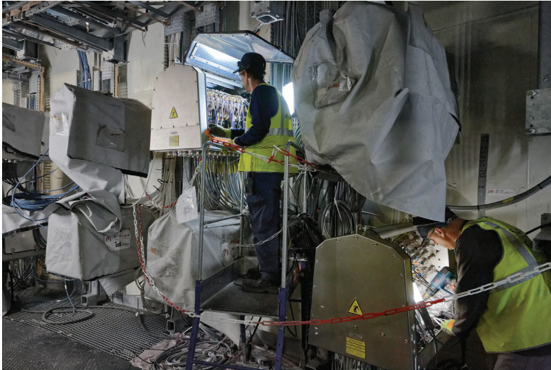
Figure 19.2. Operators inspecting electrical cables in the Flamanville 3 EPR. Alexis Morin/IRSN Media Library.
